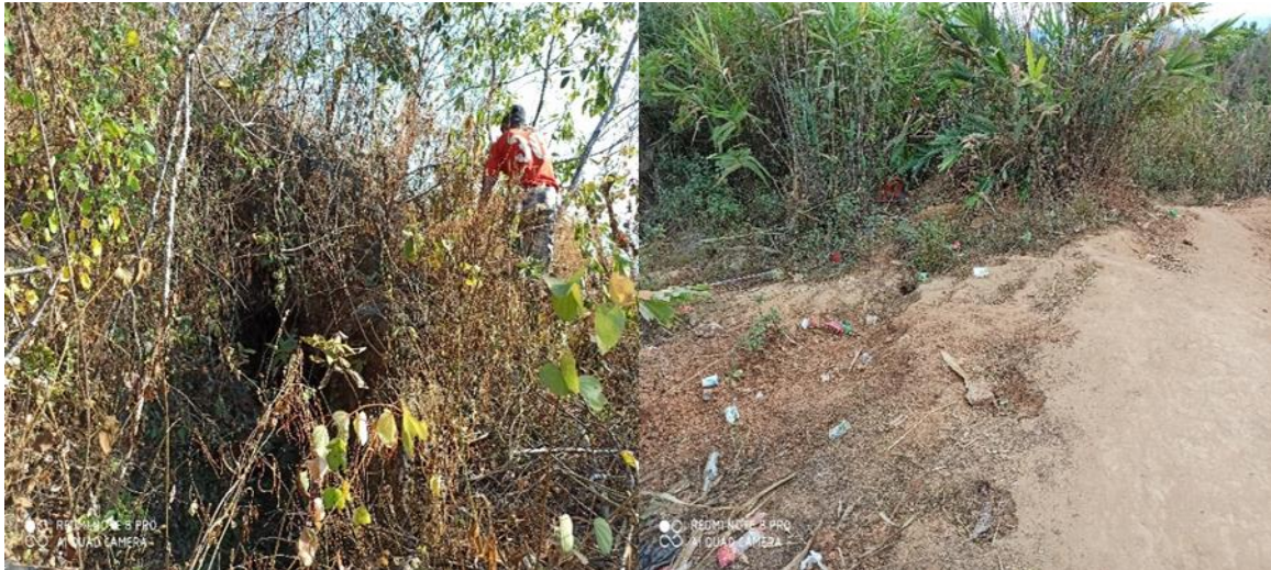
Figure 6. Open crack in site No.6 (Left) and step crack in site No.7
