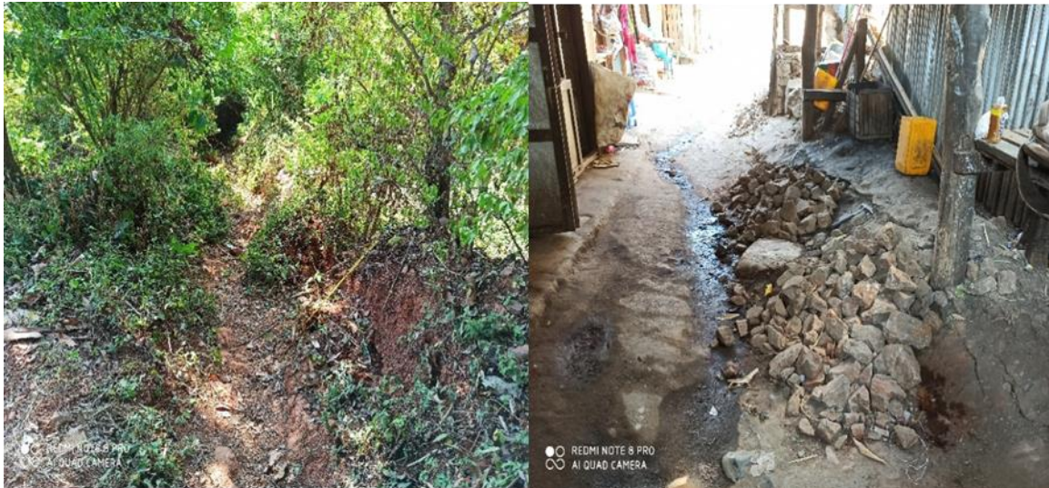
Figure 9. Step cracks in site No.9 (left) and site No.10 (right)
