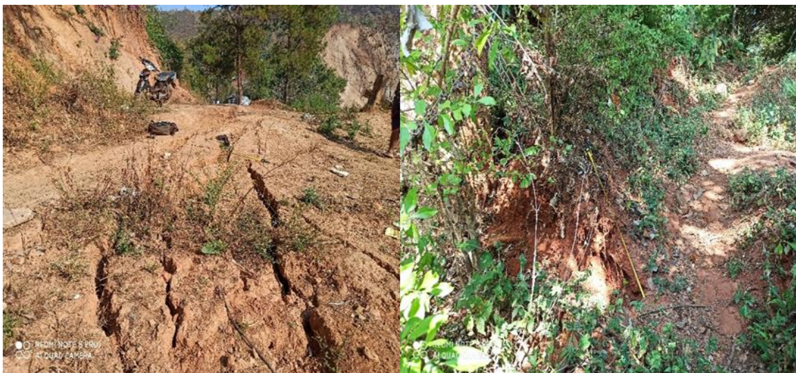
Figure 8. Step cracks in site No.9
