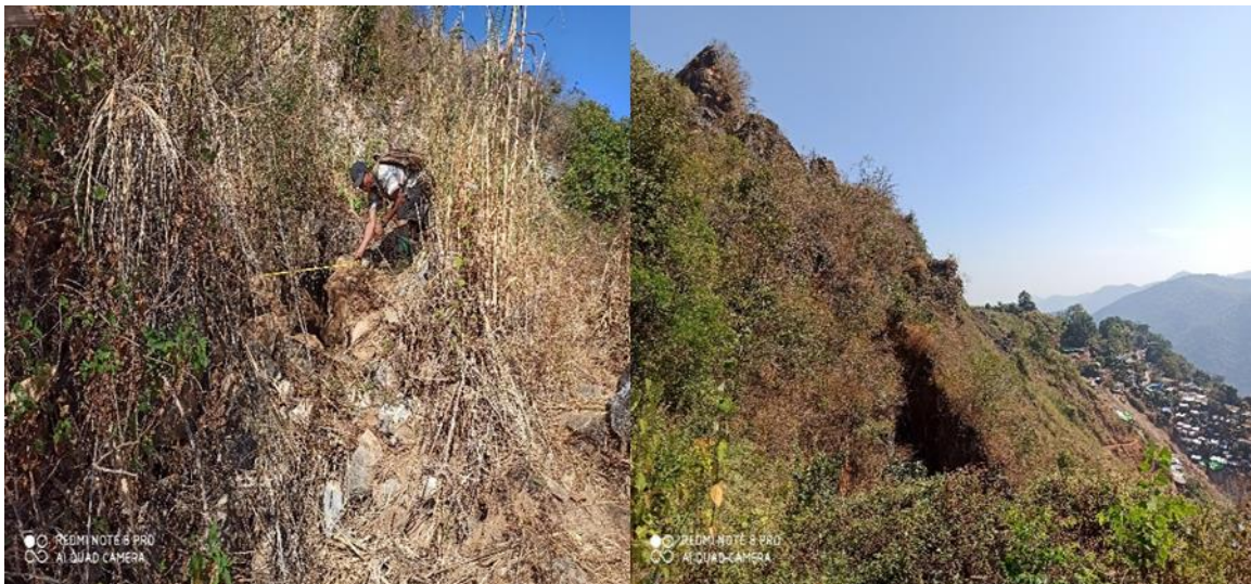
Figure 4. Step crack in site No.3 (left) and open crack in site No.4 (right)
