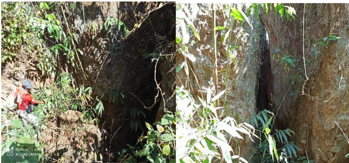
Figure 5. Open cracks in site No.5
