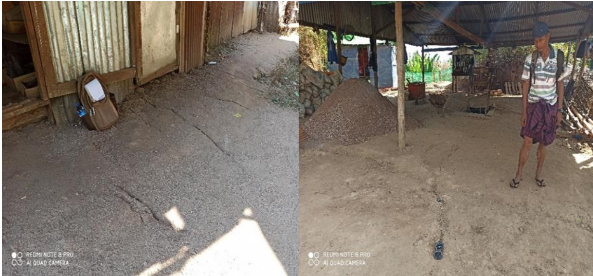
Figure 3. Tensile cracks in site No.1 (left) and site No.2 (right)
