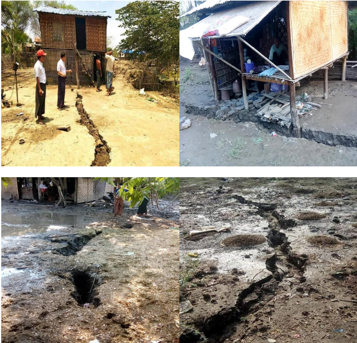
Figure 3. Some earth fissures photos reported on the social media Facebook
